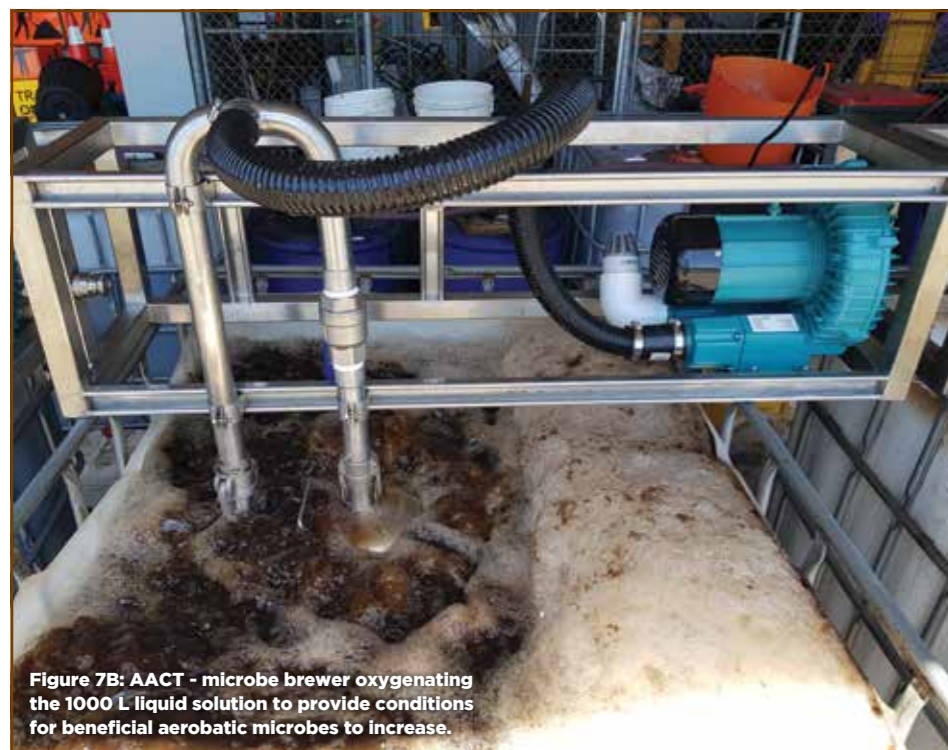
Figure 7A: G.U.F - PHC - preparation centre at the Adelaide Nursery. AACT 3 x 1000L mobile brew operation.
